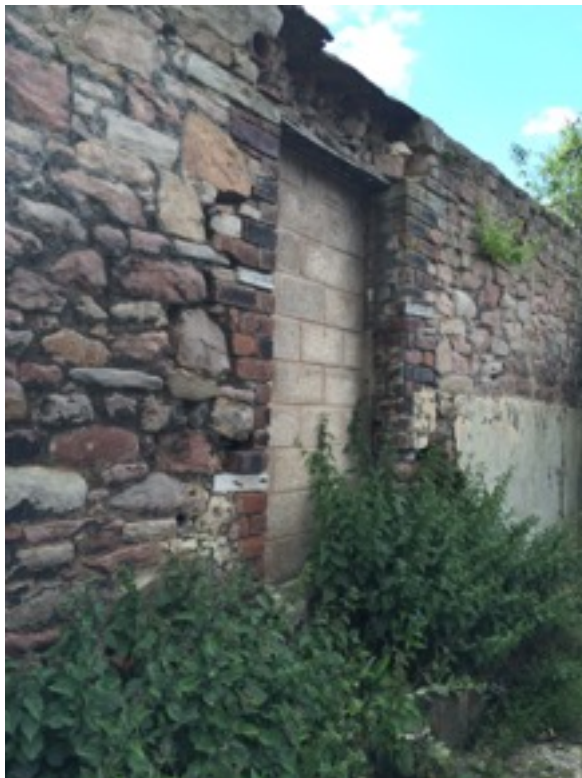
Door to north end of site: to be opened up and a timber gate put in its place.
