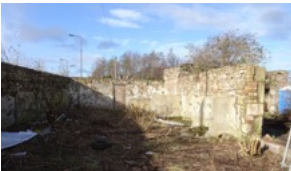
Current view within pigsty with chapel structure to right just beyond wall
