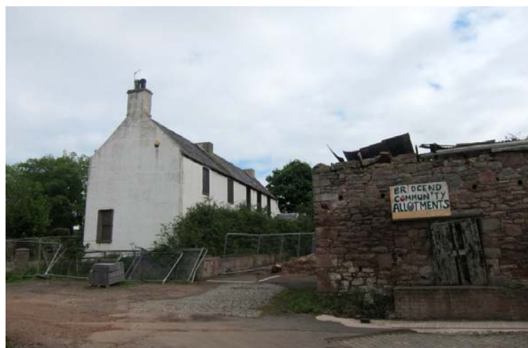
Figure 17: Current condition of the Bridgend Farmhouse
